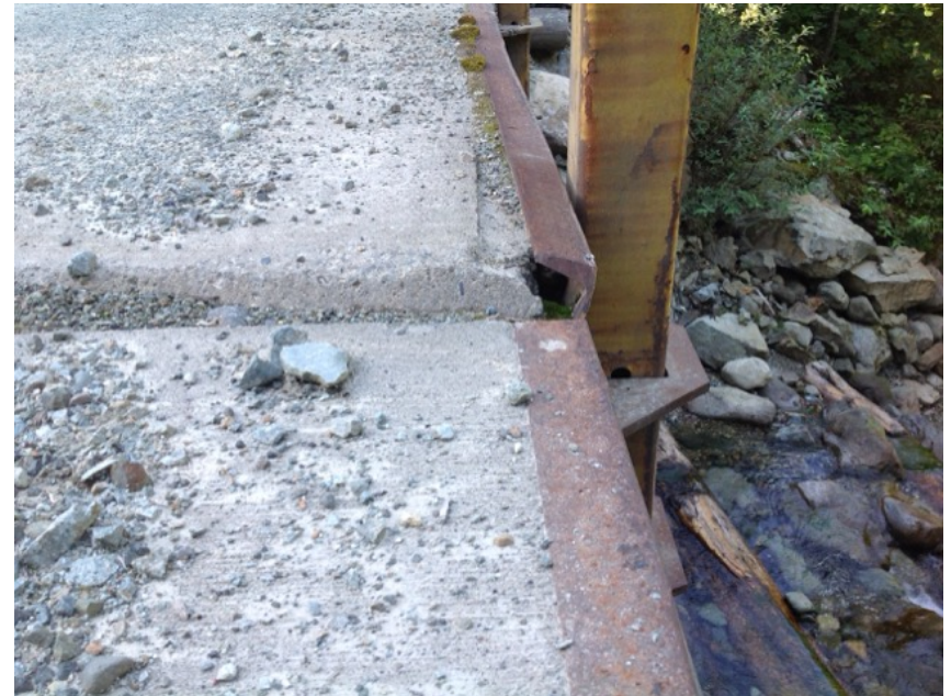
minor damage to panel
