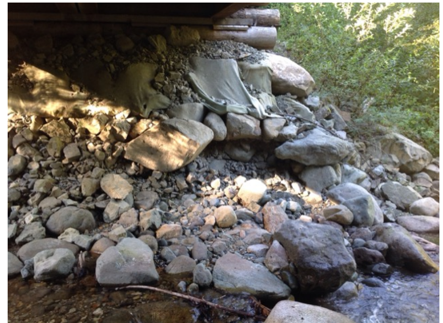
downstream left bank riprap scour
